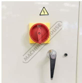
Main Isolation Switch
