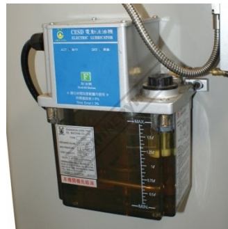
Automatic oil lubrication pump and reservoir
