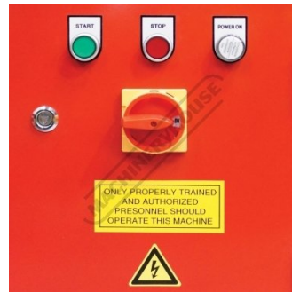
Control Panel Switches
