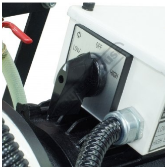
Main Power Switch
